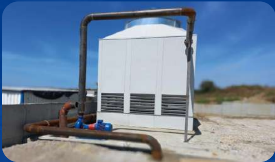
Water Cooling Tower and Pipes
